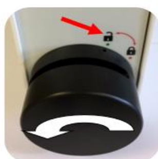
Open and unlocked protective casing (does not seal)
